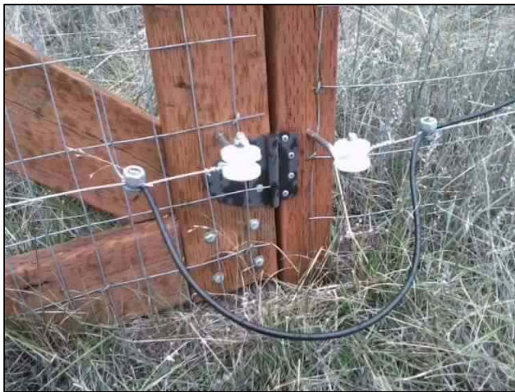
Figure 5. Black-colored insulated electric fence wire, 12-gauge. Used here to connect the electrified lines of a gate to the main electrified lines on the fence.
